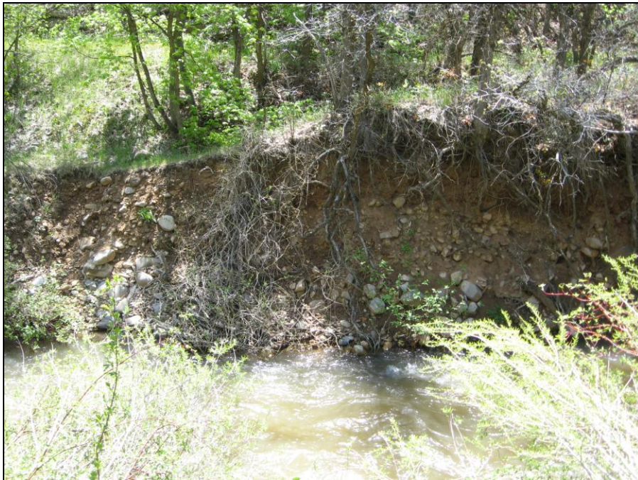
Figure 5-26: Stream Bank Erosion
