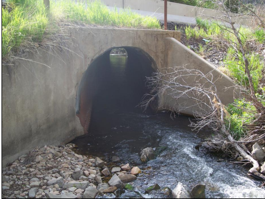
Figure 4-12: Inlet of Backwatered Culvert #3
