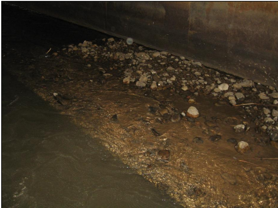
Figure 5-14: Fish Baffles Filled in With Sediment
