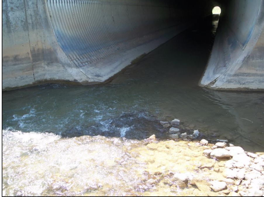
Figure 4-10: Inlet of Backwatered Culvert #2
