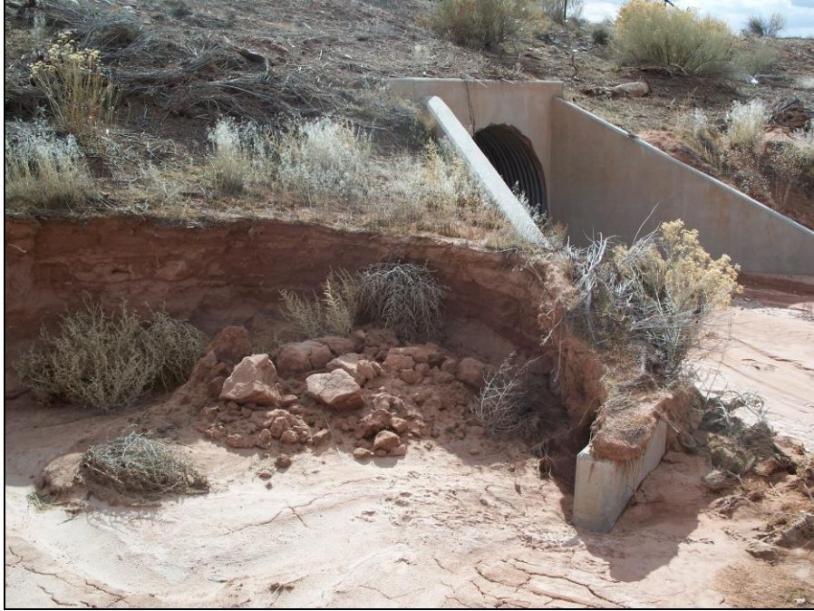
Figure 5-25: Erosion Behind Wingwall
