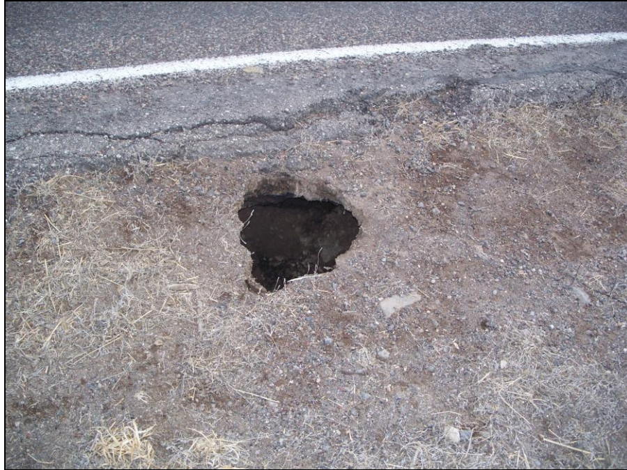
Figure 5-28: Possible Road-Side Erosion Associated with Figure 5-27
