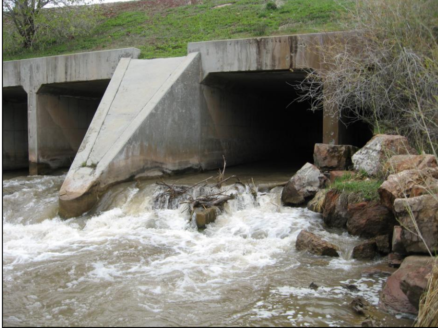
Figure 5-17: Debris Pile at Culvert Outlet
