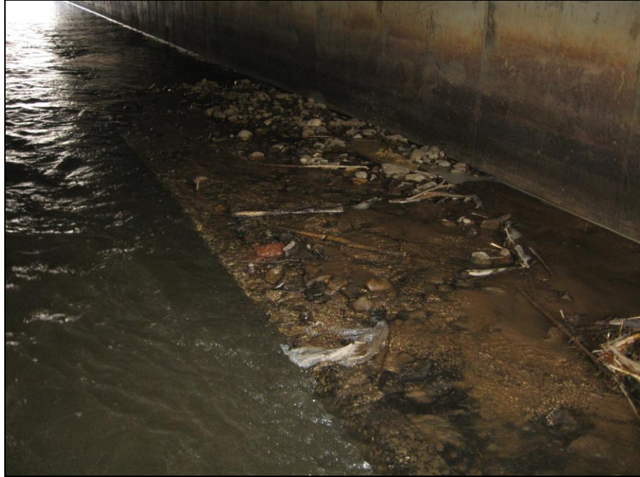
Figure 6-22: Close-up of Sediment Filled Section of Fish Baffles in Diamond Fork #2 Culvert
