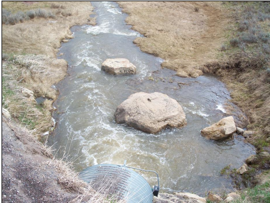
Figure 5-20: Large Boulders Downstream of a Culvert Outlet
