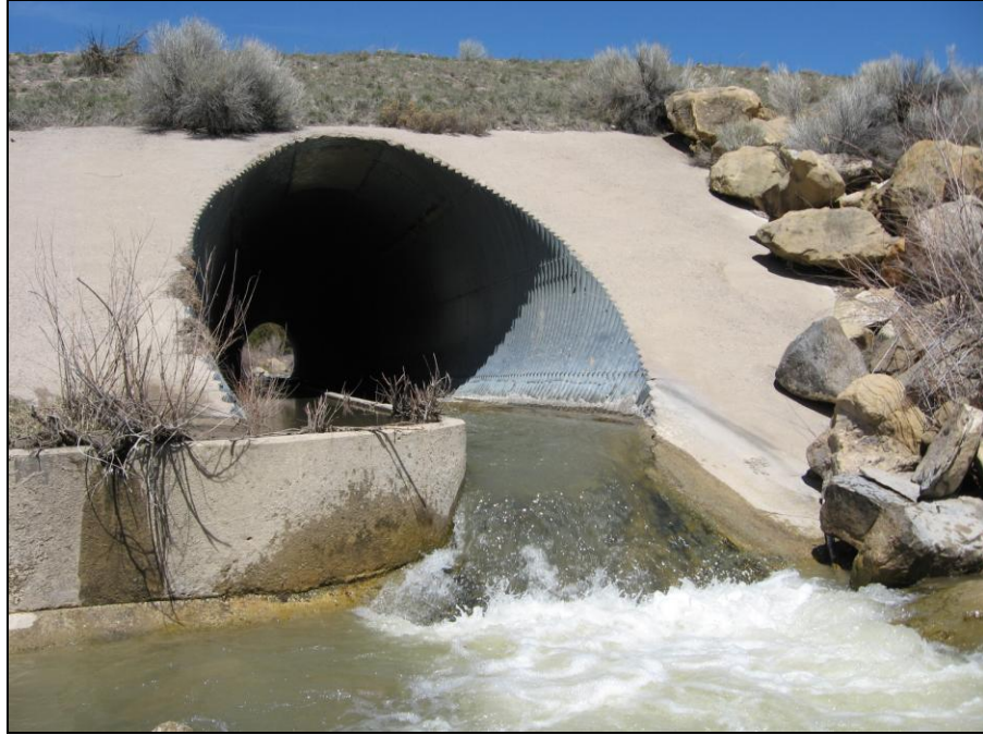
Figure 6-24: Salina Creek Outlet and Wildlife Trail Looking Upstream
