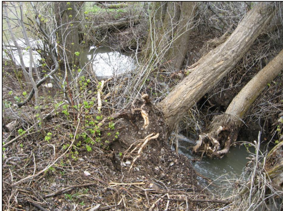
Figure 5-9: Debris Dam Causing Backwater Conditions
