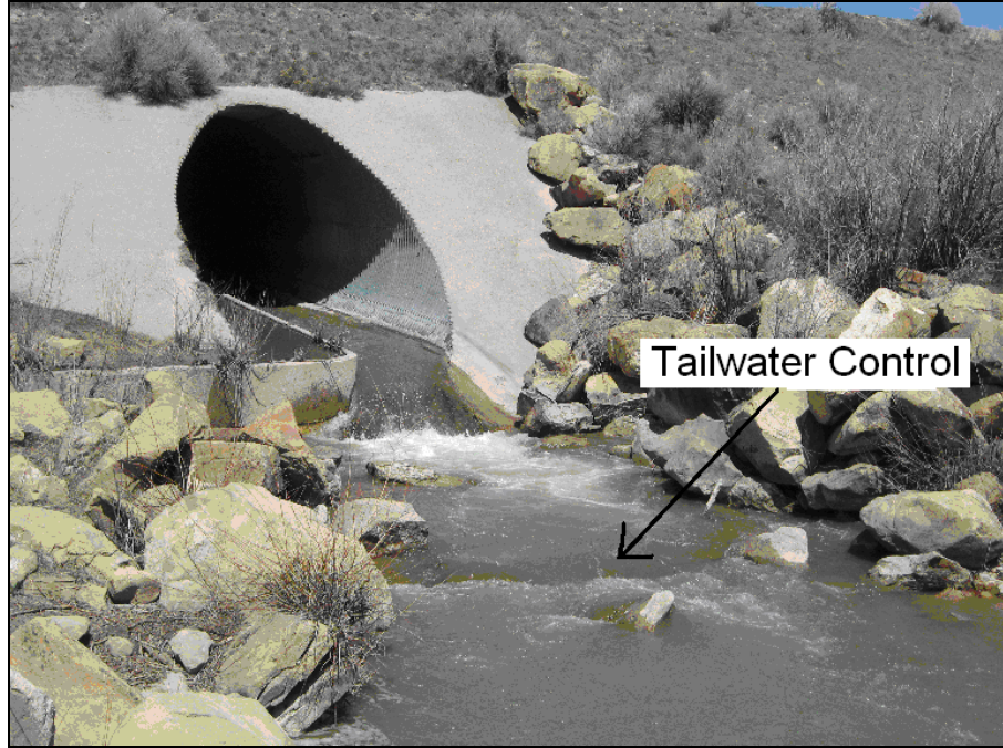
Figure 5-5: Outlet and Tailwater Control Photo
