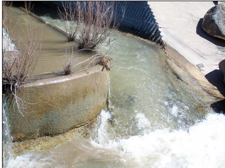
Figure 5-6: Photo of Discharge at Outlet Invert
