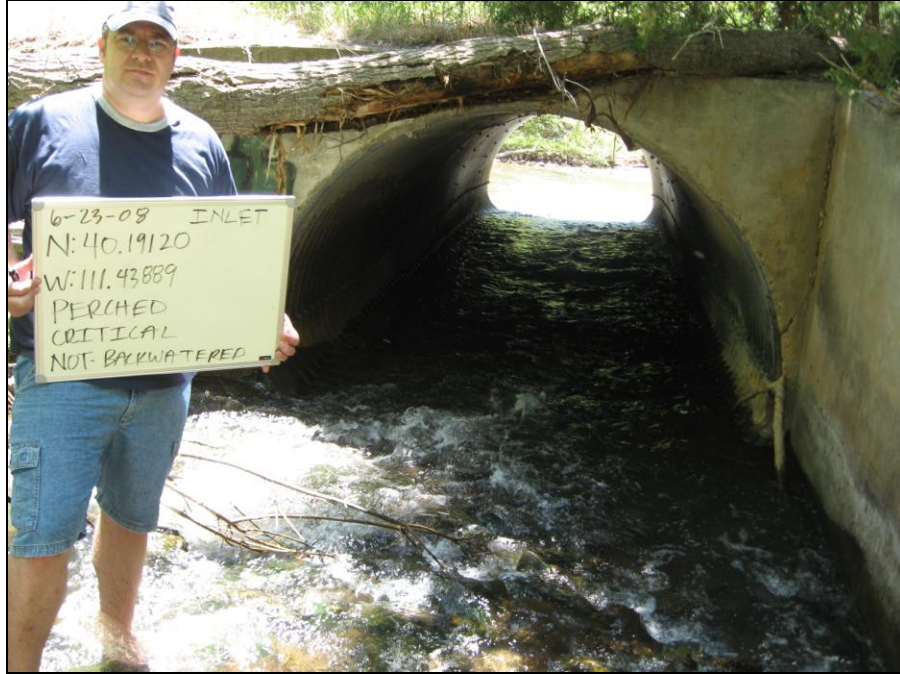
Figure 4-3: Hydraulic Evaluation Photo Taken at the Inlet
