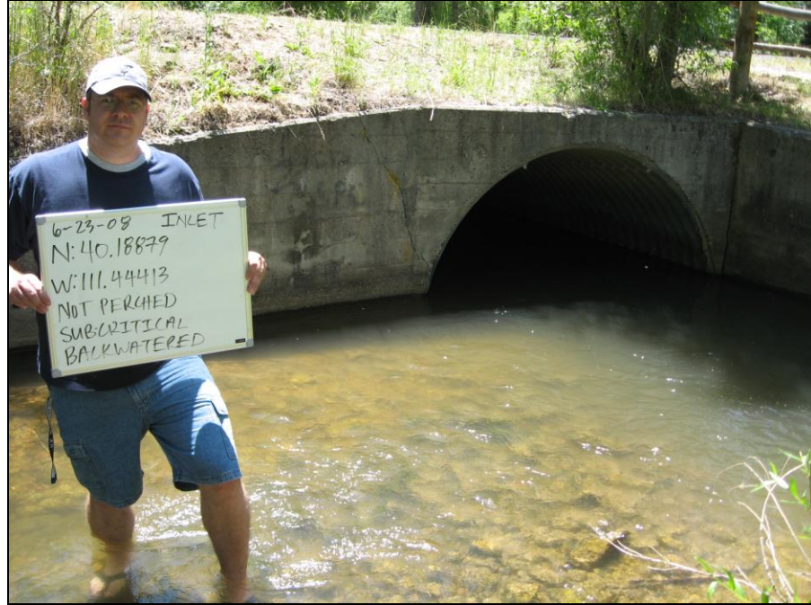
Figure 4-1: Hydraulic Evaluation Photo Taken at the Inlet
