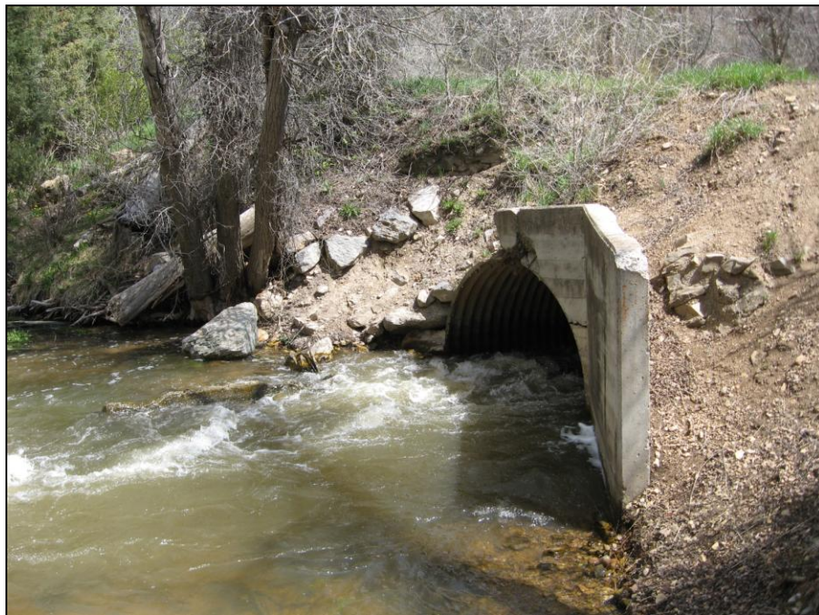
Figure 5-29: Stream Bank Erosion and Failure of a Culvert Headwall
